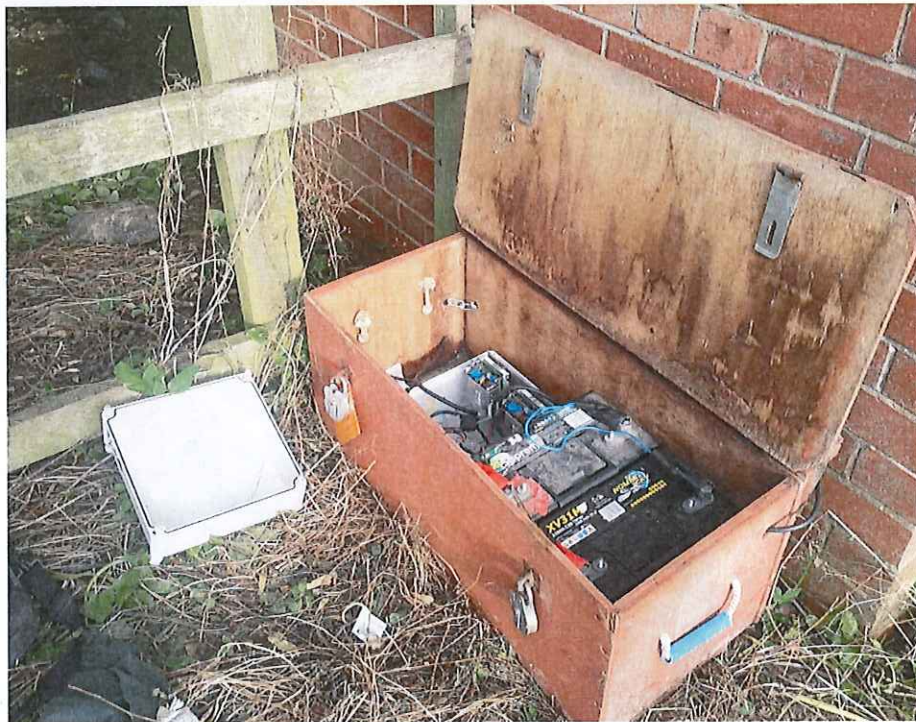
Figure 2.2: Weather-proof box housing Deerness PIT logging equipment and batteries. Photograph taken on 24/09/2014.
