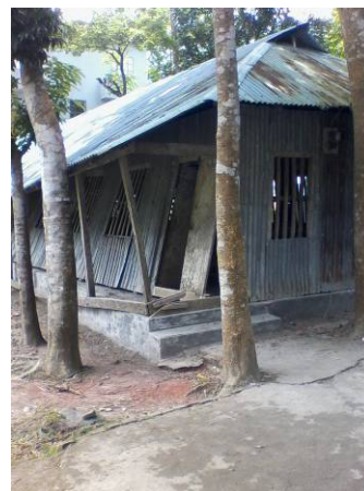
Damage in the Cyclone Mahasen in 2013
