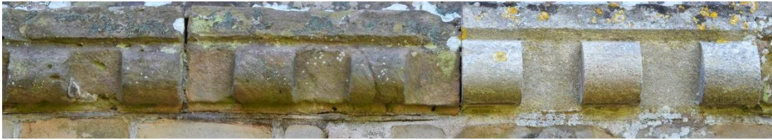
Fig. 2m. Exterior stringcourse (original on the left and renewed on the right), St Mary the Virgin, Upleadon, Gloucestershire.
