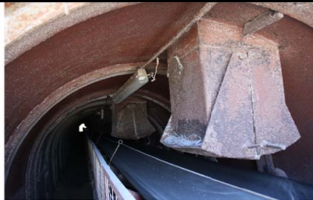
Shutters in the tunnel roof allow material to fall onto a moving belt by gravitational forces (opening size can be adjusted to modify rate of flow)
