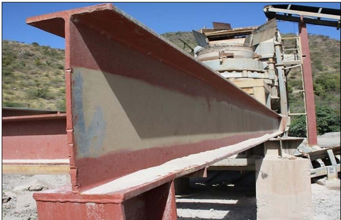
Figure 3.18 Dust accumulated on base of the girder of the processor at Little Bay, Montserrat, West Indies.
