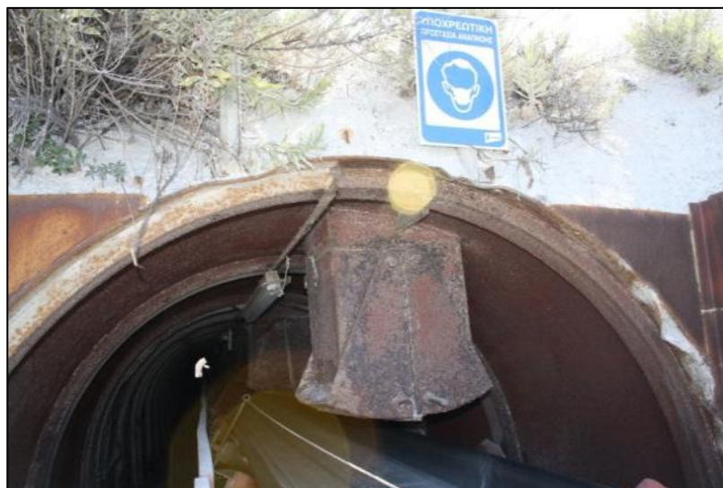
Figure 6.18 Notice to wear respiratory protection at entrance to tunnel in LAVA pumice quarry, Yali.
