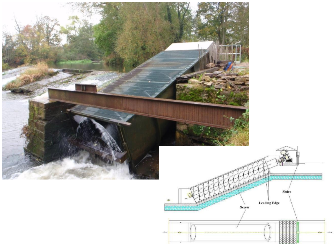
Figure 2.2 Hydraulic screw turbine in place at Howsham Mill and schematic of Archimedes screw turbine shown from the side and above (inset; MannPower Consulting).
