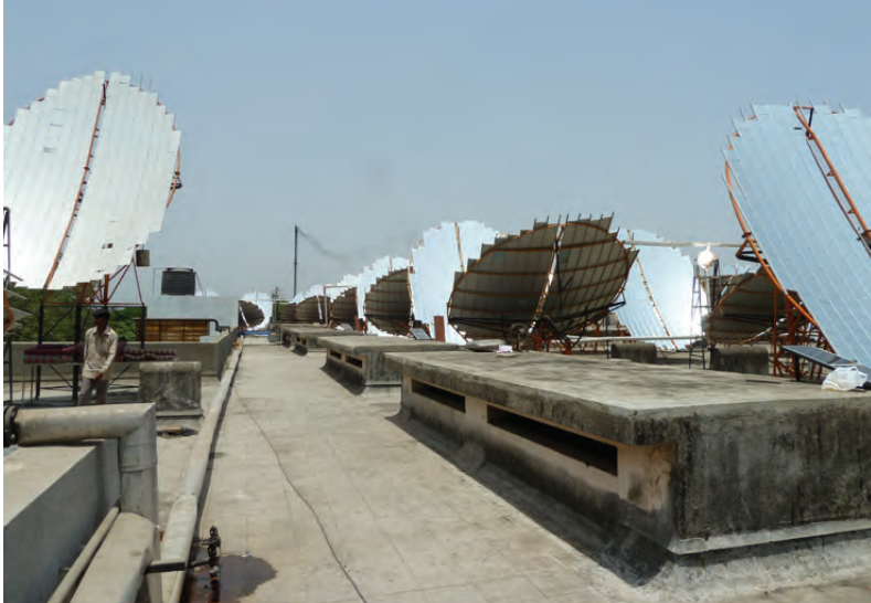
Figure 5.4: Solar parabolas for air conditioning at Thane's main public hospital.
