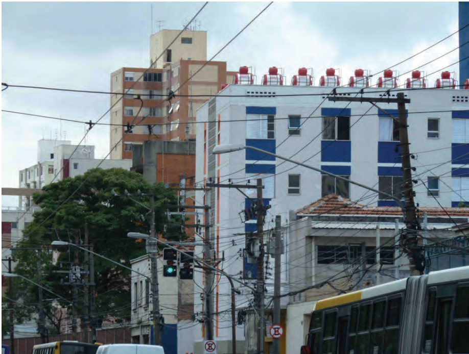
Figure 4.8: SHW systems on the roof of a residential tower completed in 2011 by the CDHU in central São Paulo (Case study 3).
