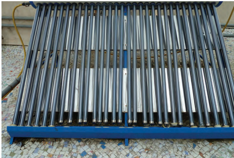
Figure 7.10: Malfunctioning SHW systems in social housing, Thane.
