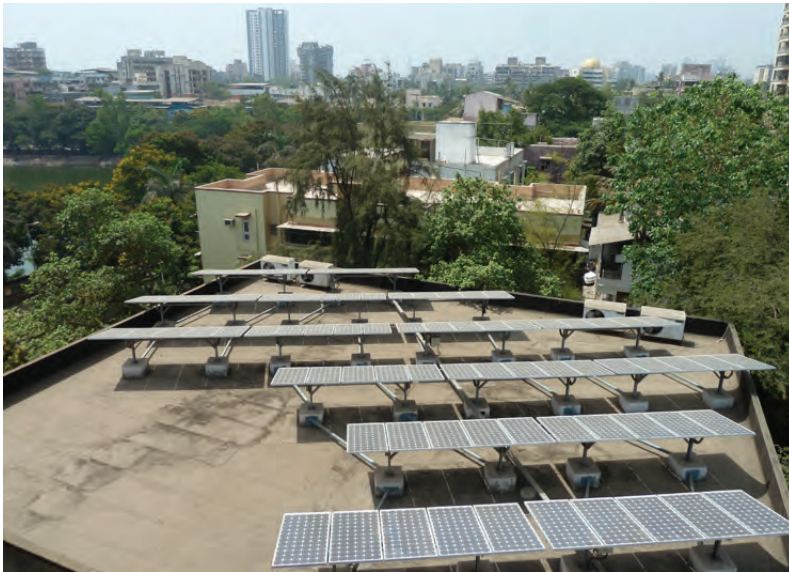
Figure 5.5: Solar PVs on the main building of the Thane Municipal Corporation.
