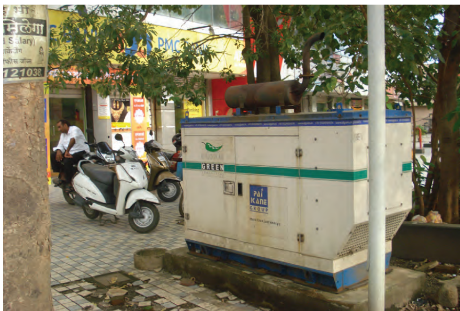
Figure 2.3: Private diesel generator for electricity provision, Thane.
